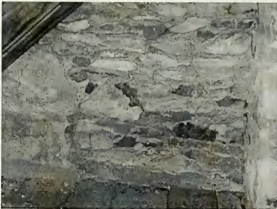
Figure 35 North Gable-End Wall in Attic of the Center Section of the Main House, 2002
